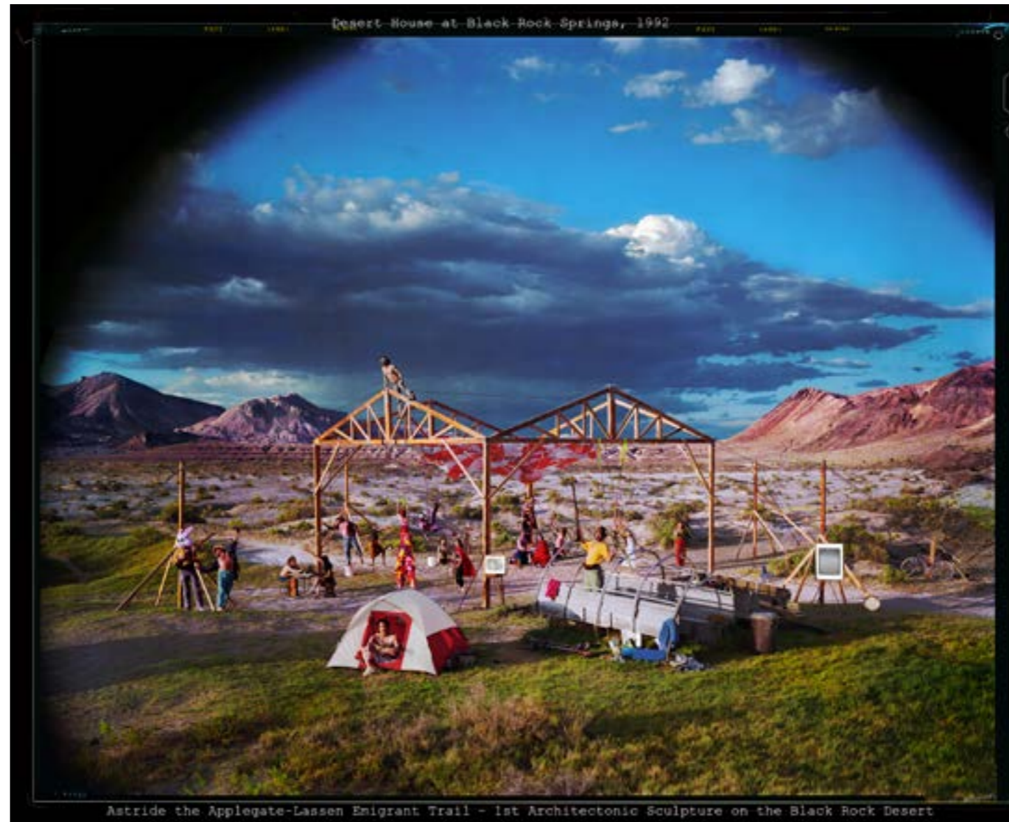
Desert House at Black Rock Springs – 1st Architectonic Sculpture on the Black Rock, 1992. Photo credit: William Binzen.
